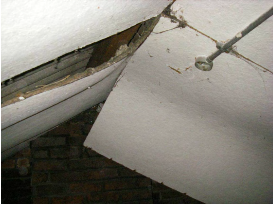
Plate C.7: Lining of roof of Building 1 damaged by damp
